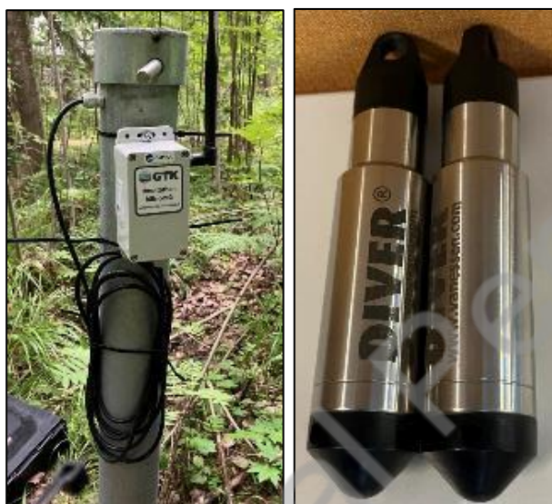
Figure 18. Left: Installed remote access groundwater sensor in the groundwater observation well at the VECTES site. Right: Van Essen Diver sensors.
