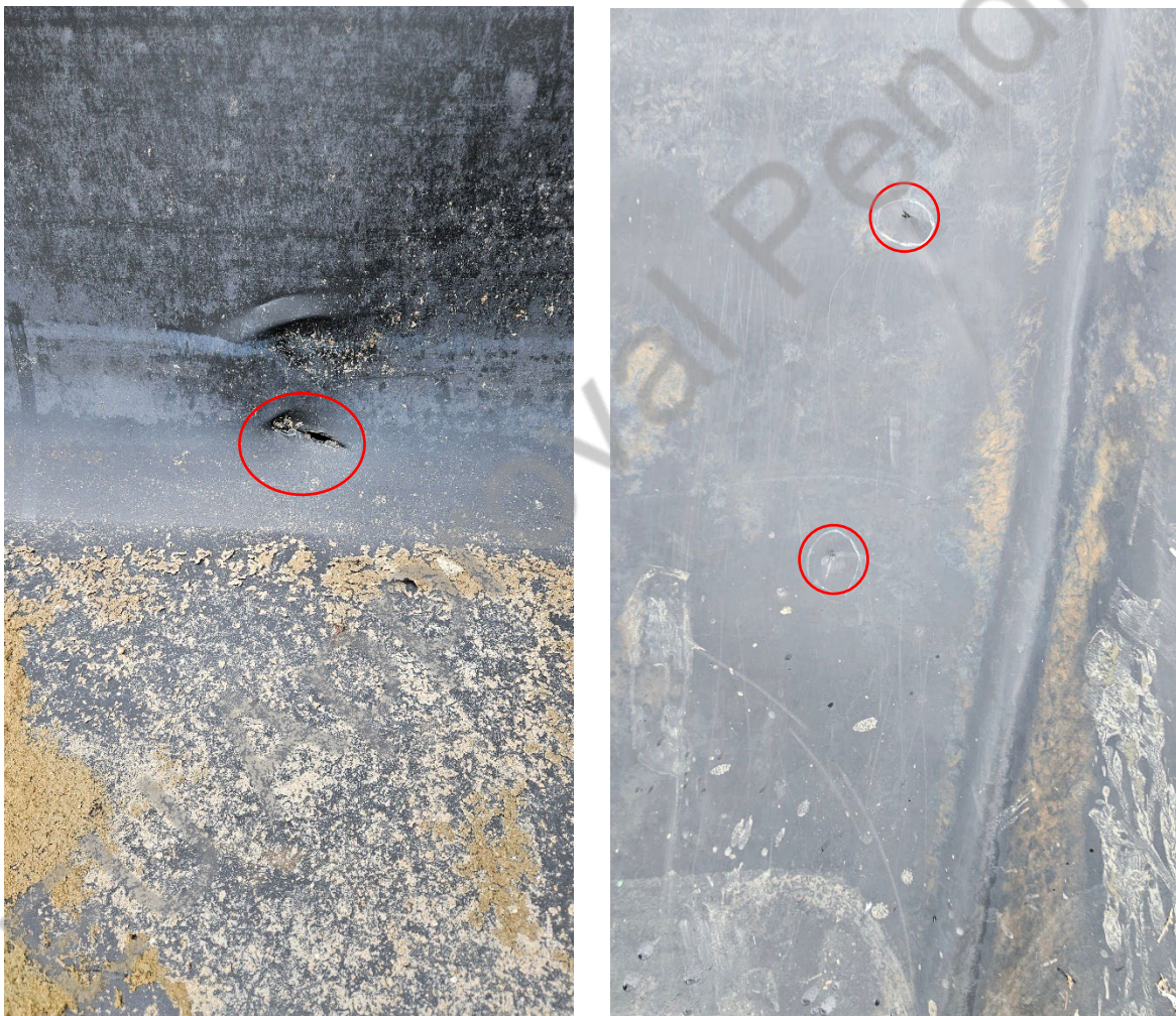
Figure 53: Holes in a sealing sheet of the Basins (Planungsgruppe M+M AG, 2024a).
