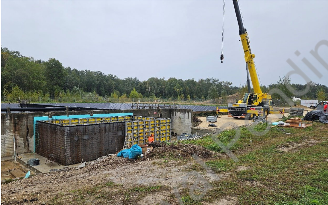
Figure 54: Hydraulic control room: Formwork of the floor plate and exterior walls (Planungsgruppe M+M AG, 2024a).
