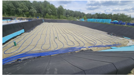
Figure 10: Installation of charging and discharging heat exchangers in basin C with the configuration H3.
